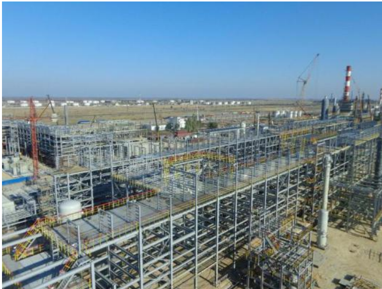
Figure 5 : Volgograd Deep Conversion Project in Russia
